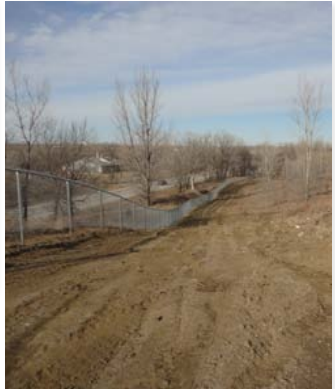
Though not steep, the grade on this fenceline trail is too long making the tread watershed very large. This area is subject to high-intensity thunderstorms, so the erosion risk here is high.
