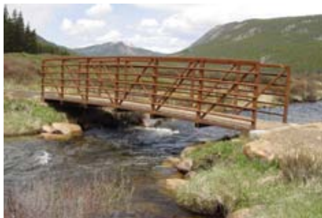
This prefabricated steel bridge is durable and has a natural appearance in this open setting.
