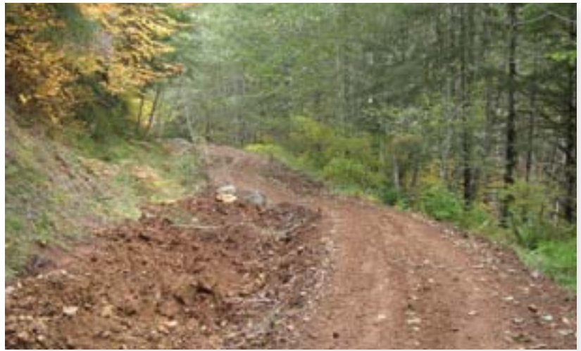
Steep, unstable ground forced the trail to stay on the existing roadbed, but the designer has created a nice sinuous flow. Ripping the unused portion of the road increases water absorption and decreases the tread watershed.
