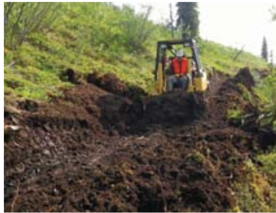
Once pioneered, the next passes build the cuts and fills to shape the trail prism and establish grade.
