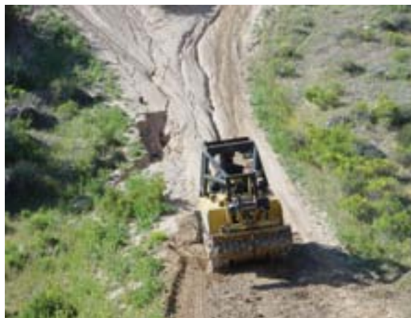
This trail is in obvious need of reconstruction. The tread watershed is too big and too much water is draining at this point.
