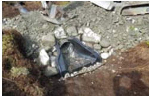
A flared inlet and headwall are being added to this culvert to help funnel the water into the inlet. Though a small diameter culvert like this may be adequate to handle the flow of water, it is very hard to keep cleaned out.
