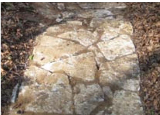
This hardening installation is composed of chunks of sidewalk that was headed for the landfill. Being heavy and angular, the pieces should key together very well. Notice that they have been embedded so that the edges are contained by the natural soil.
