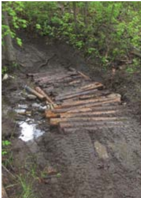
This poorly crafted installation was thrown together during an exceptionally wet spring. It is too short, too narrow, and some of the logs are floating. Some ditching should have been done to help drain the water better. This is a good example of the issues usually associated with corduroy: poor patch jobs that don't address the problem and usually degrade into a hazardous situation.
