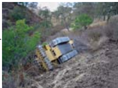
Equipment can find its way into precarious positions.
