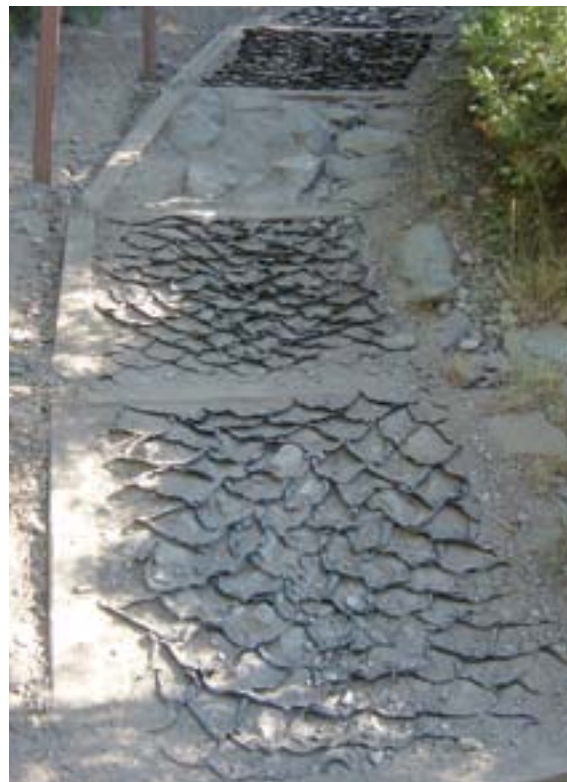
This is an excellent example of boxing in the trail hardening to provide lateral and longitudinal support. Unfortunately, the cover over this geocell has been lost and the structure is rapidly degrading. The large cobble rock in the center section is actually holding up better.
