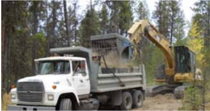
A clamshell bucket is also very handy for plucking trees, stumps, or rocks. This one has a built-in grizzly that allows dirt and smaller rocks to fall through.
