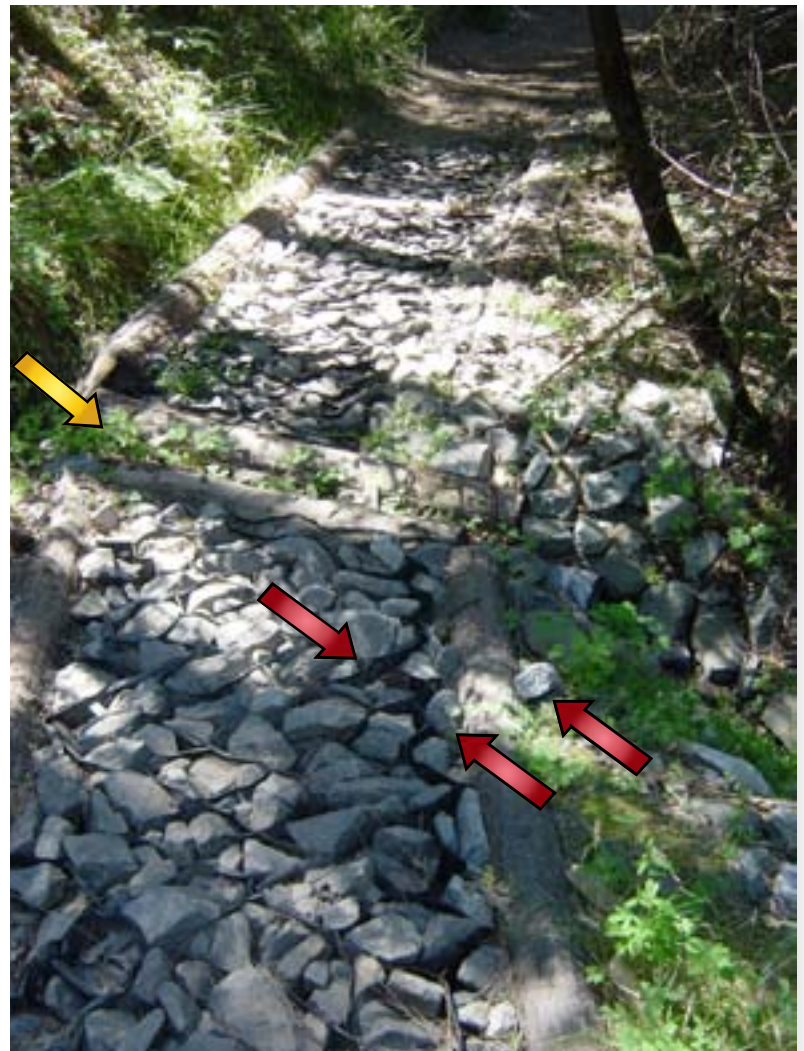
This is an excellent example of a trail hardening installation that will likely fail. On the plus side, the material is framed into sections which help prevent movement. The gap between these two sections (yellow arrow) serves as a log culvert. On the minus side, this cobble surface is rough to ride on and the rotation action of the tires will displace the rocks out of the Geocell (red arrow) and the exposed cells will start to break down. The life and functionality of this structure could have been extended if it had been covered with a layer of well-graded aggregate.
