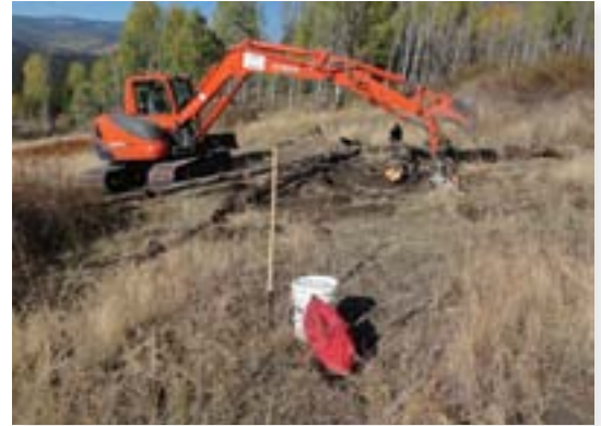
An excavator places debris and installs logs in a herringbone pattern to close off hillclimbs on a sensitive grassland. Note the hand-seeder and bucket of seed ready for immediate application.
