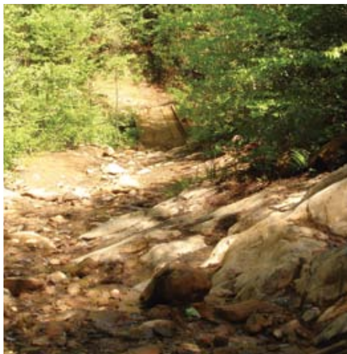
This is a common, but poor bridge approach. This long grade has no drain. All of the water and sediment will be deposited directly into the creek. Vehicles trying to brake going down or accelerate going up will churn up more soil that will also end up in the creek. Old roads are often used for bridge access because they are existing and provide a means to get equipment and materials into the bridge site. This is okay, but using the road as a trail afterward isn't. A properly designed trail should be located and constructed and the old road closed.
