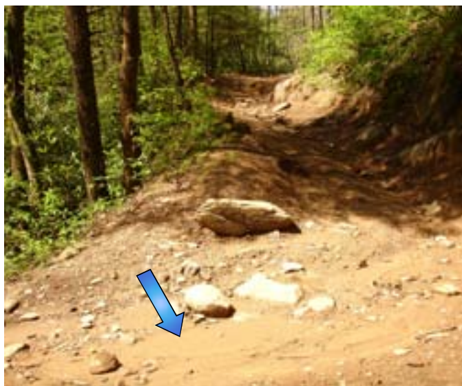
The trail turns and dives down to the bridge at a steep non-sustainable grade. Look at the amount of sediment (arrow) that is getting ready to be flushed down to the bridge.
