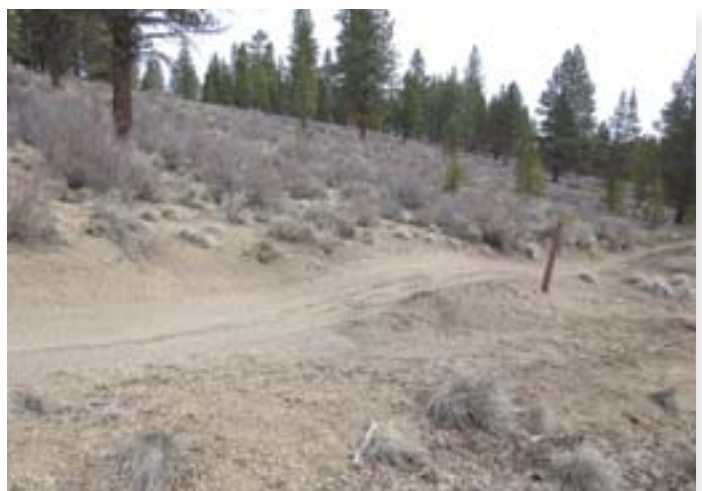
Though this dip rides nicely, it wasn't constructed with enough elevation difference from the sag to the crest. Due to the soft, non-cohesive soils, displacement from a few motorcycles has already created a rut deep enough for the rolling dip to fail.
