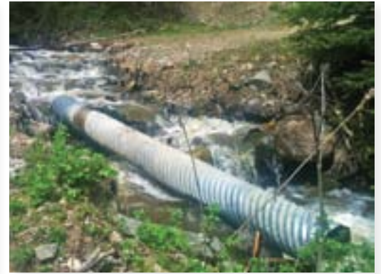
When culverts are undersized, the results can be disastrous and expensive. Spend the money up front to do it right the first time.
