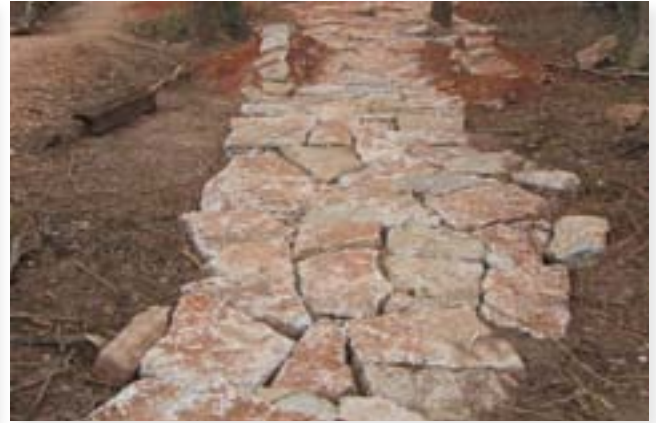
These rock slabs are well-placed and keyed together, but they lack confinement. Rotational and centrifugal forces will gradually displace them.
