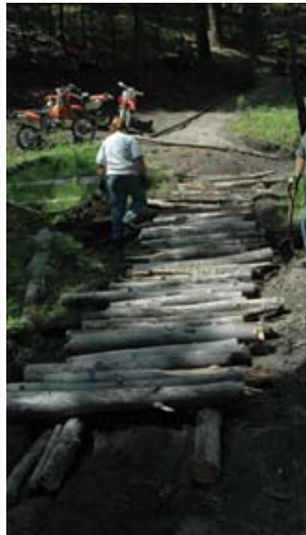
Corduroy anchored onto stringers will last longer and create a more stable tread. This is an example of a poor quality installation. The stringers already show signs of rot and the corduroy logs should have been cut into even lengths.
