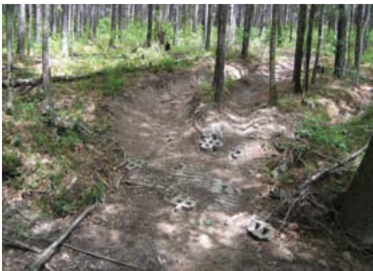
The results of a poor installation: broken pavers, two eroded trenches instead of one, risk, resource impacts, and a mess.
