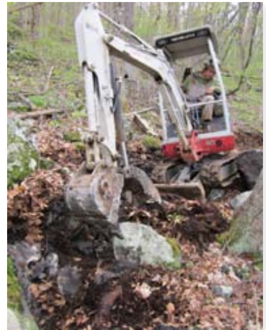
A dozer can push through a rock pile like this and some of the rocks may roll down the hill. An excavator can create a bed for the rocks and carefully place each one. Rocks like this can be used to support the trail tread or used as anchors or chokes for the trail which will enhance the trail's aesthetics and the rider experience.
