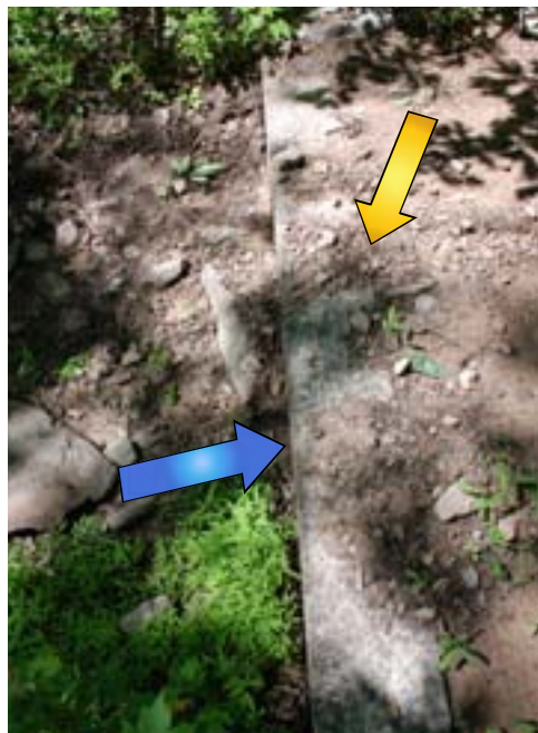
This treated timber waterbar provides a formidable obstacle from below (blue arrow) and being full of sediment, it provides ineffective drainage (yellow arrow). The issue: the tread watershed is too large. Poor soils cannot sustain this grade that is too steep for too long. The solution: relocation.
