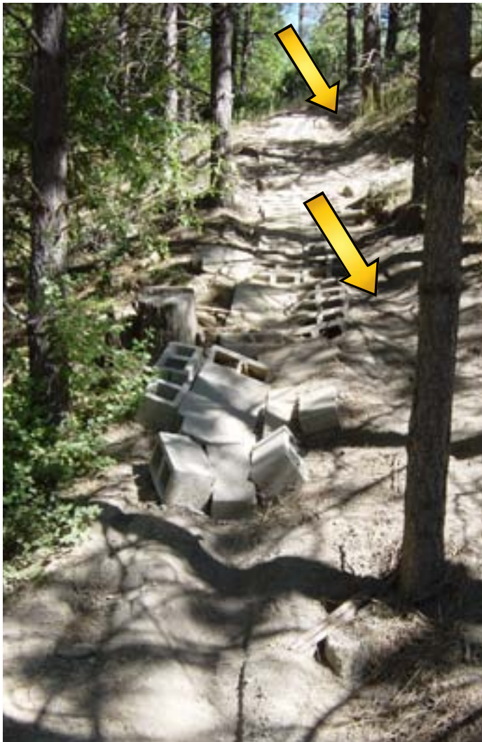
Poor bedding + no containment + movement = failure. You can see (arrows) where riders are going up the right side to avoid this installation.
