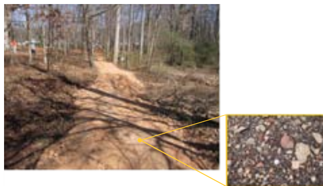
This hardening installation is another recycling project. A brick and concrete high school was being torn down and was headed for the landfill, but a heads-up project planner thought to grind it up and try it for trail hardening. The material was free, it worked, and it set up like concrete due to a good mix of particle sizes. This was a win-win for the project, the community, and the environment.
