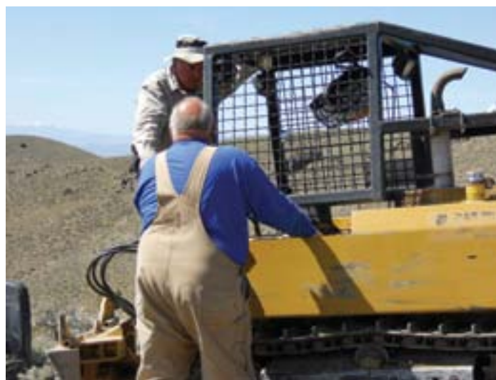
Equipment down time is project down time. The project manager and operator discuss the source of and remedy for a hydraulic leak.
