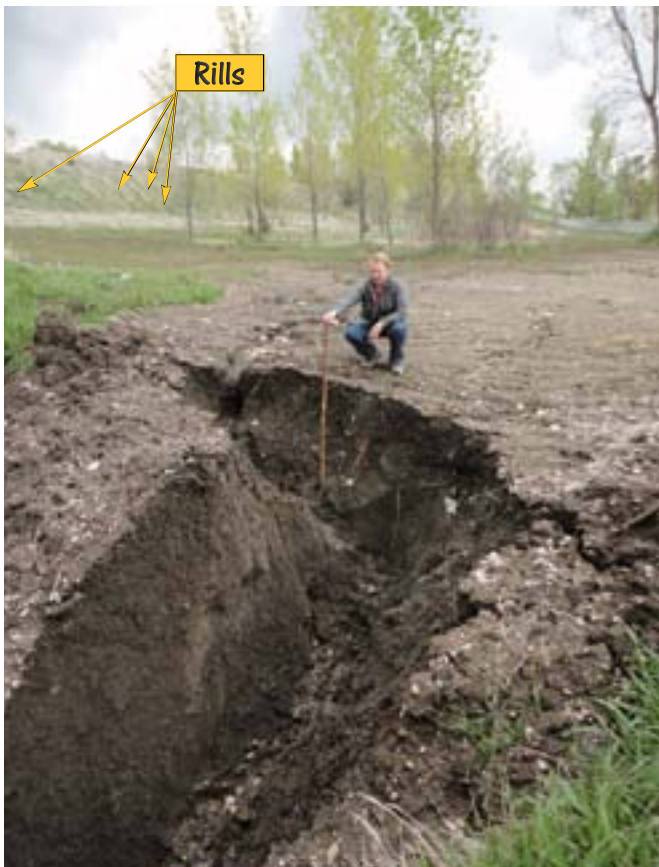
This is a view of the bottom of a large tread watershed. The soils on this site are very poor. When the spring storms started, so did the erosion. Though grassed in, look at the rills on the slope that are feeding water to this drainage point.
