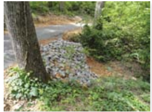
A blanket of cobble rock at the drain point of this trail protects the fillslope from scour and erosion. This protection is especially important where there is the potential for high volume and high velocity water flows.
