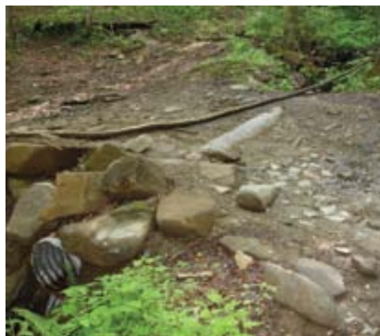
The top of this culvert has been damaged and will eventually break which compromises the integrity of the structure and increases agency risk.
