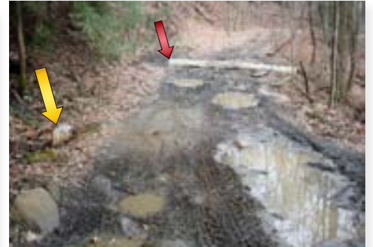
The first culvert (yellow arrow) was properly installed in the drainage. The second culvert was added later possibly to drain a spring but was not installed properly due to rocky ground. Manage your risk. The second culvert does nothing but create a safety hazard and an opportunity to ruin what was a good section of culvert. A side ditch draining into the first culvert may have been a better solution here.
