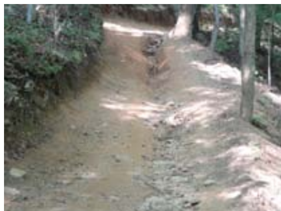
A sight like this is commonplace, but it represents a water management issue. It's important for maintenance personnel to recognize that it is an issue, determine the cause, and identify the solution.
