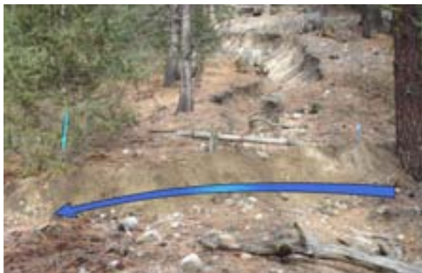
Before rehab efforts could begin on this heavily eroded trail, the source of the water had to be diverted away by ditching it into the natural drainage courses.
