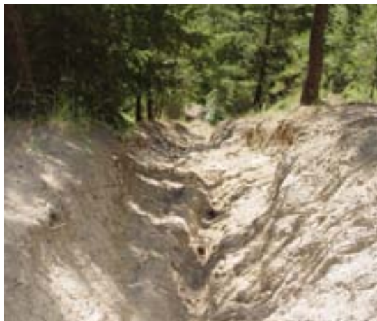
This severe erosion occurred below a road drainage point after a high-intensity thunderstorm. The sediment carried all the way to a sensitive creek below.
