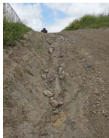
Due to a lack of training or awareness, maintenance personnel have bladed out the rolling dip at the top of this steep hill allowing water to run down and erode the slope.
