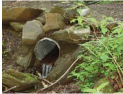
There are drawbacks, but culverts allow water to drain under the trail and keep the tread dry.
