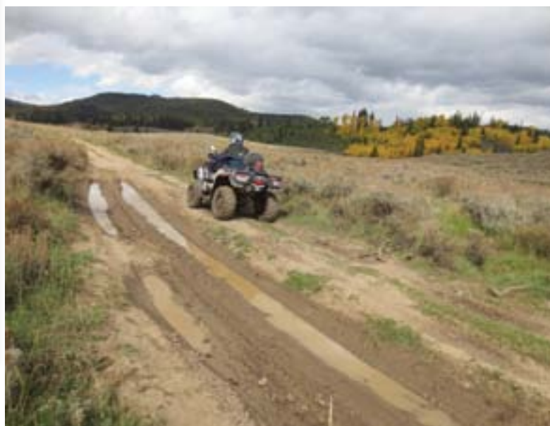
When constructed, this low spot was outsloped to drain water. Through compaction, displacement, and lack of maintenance, the trail bed is now lower than the ground on the downhill side. So the water ponds up in the trail which is causing trail braiding. The trail now requires reconstruction and armoring with rock to help maintain the shape and provide additional bearing when it is wet.
