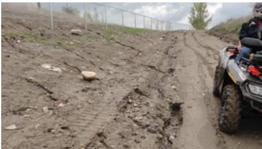
Notice the rills of water draining down the slope and into this trail. Notice also how quickly the rill down the edge of the trail deepens as more water feeds into it and the water velocity increases.
