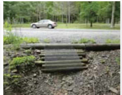
Manage parking lot drainage through design. The low point of this lot is at the trail access point so all of the water flows down the trail. Attempts to harden it will be futile and the best option is to relocate the trail access point.
