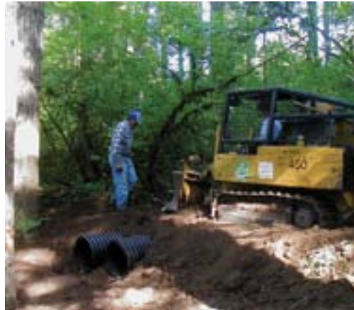
It is dry now, but this runs a lot of water in the winter. Two plastic pipes in this shallow drainage keep the trail fill low and provide a safety net to handle unusually heavy flows. Two pipes have to be carefully bedded to prevent water from running between them.
