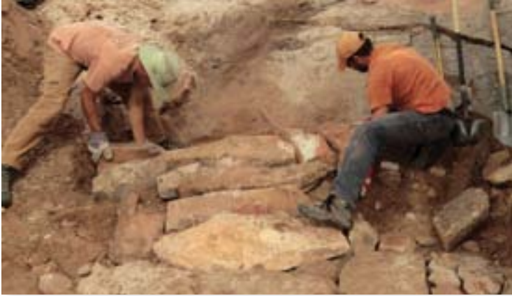
The approach to this technical step-up is being armored to prevent the step from getting higher and eventually becoming unrideable.
