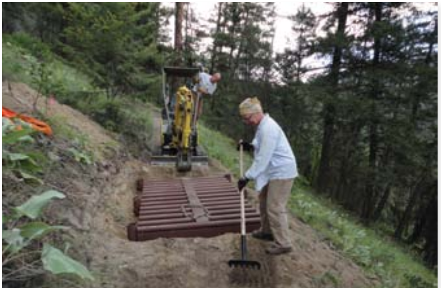
A fenceline needed to be installed to keep livestock out of a stream to protect water quality, but there were limited places to cross this trail. This site was chosen after coordinating with range and the range permittee. Water, range, and recreation all benefitted by this cooperative effort.
