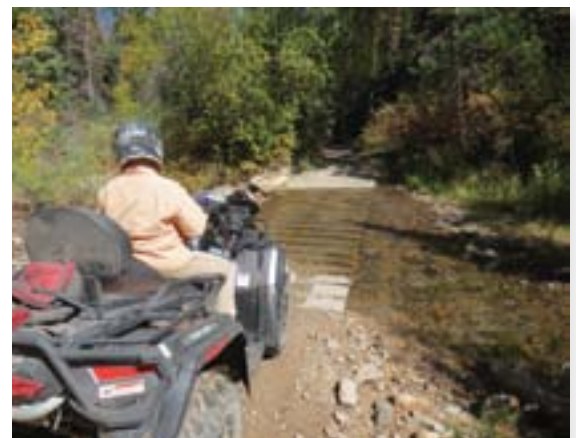
This ford is hardened with concrete boat ramp planks. These are commonly used and they work quite well.
