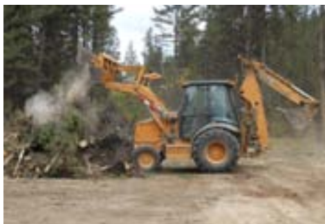
The clamshell bucket on this backhoe adds to the machine's versatility. It can scoop, load, back blade, pluck, place, and chop.
