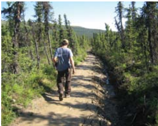
A side ditch was cut along this trail to help drain the trail tread. However, it does not have adequate cross drains so the water is running too long and too fast which has resulted in erosion. Cross drains need to be added here or the ditch lined with rock to dissipate the water's energy and protect the ditch side walls.
