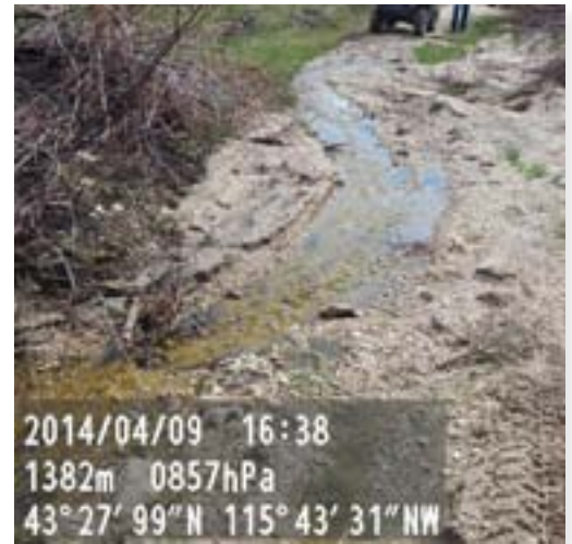
A geotagged photo documenting a water issue
