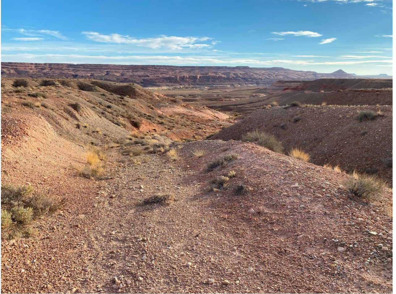
Photo 4, a view of water erosion on SD 781 in 2020.
